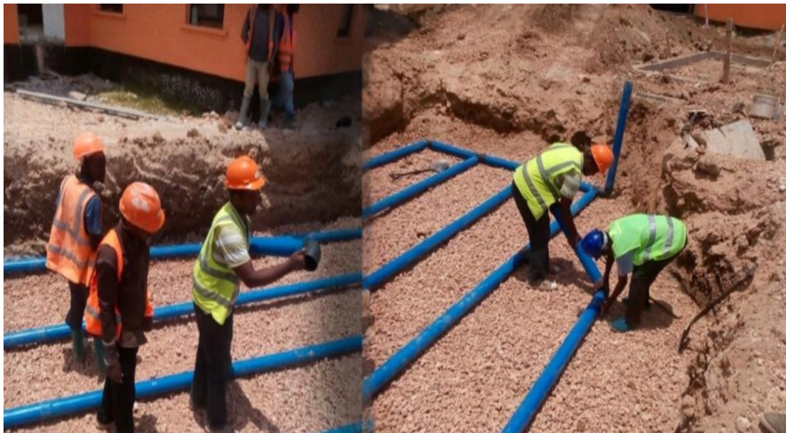
Photo 1. 2 Installation of French pipe for ground discharge of final effluents from ABR
